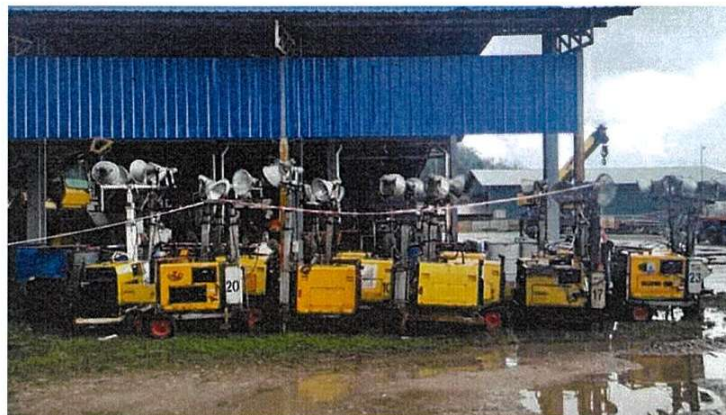
Photo 4: Portable Light Generator
